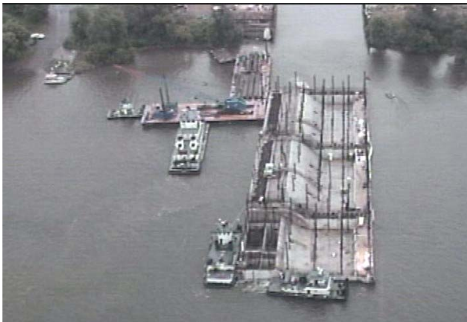
b. Float-out or launch of the first segment of the dam Figure C-10. Braddock Dam Casting Facility
