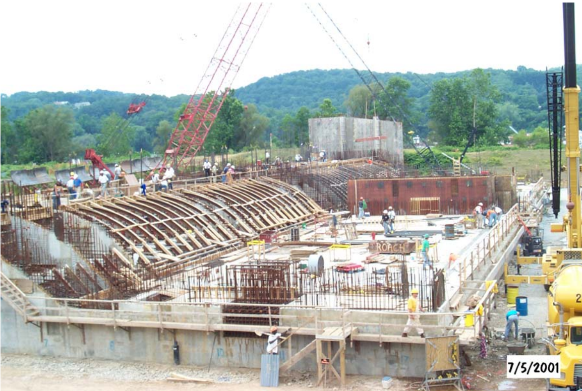
b. Construction of dam Segment 2 within the two-level casting basin Figure C-11. Assembly of float-in Braddock Dam at casting facility
