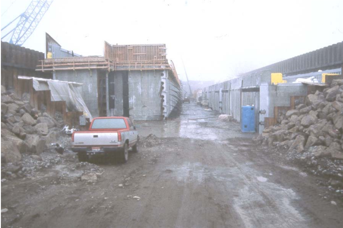
Figure C-21. Precast yard in Bordman, Oregon, for Bonneville Project. The contractor constructed a graving dock. The pontoons were fabricated, the site was flooded, and the pontoons were towed to Bonneville for installation
